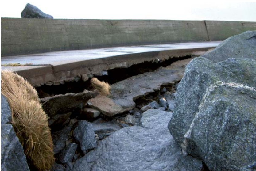
Figure 8-23 Damage under the deck and on the back side after overtopping and penetration by high waves. The convex shape of the deck and a solid concrete front contributes to preserving the shape of the deck and prevents its total failure. (Tynnes Breakwater, Værøy. Photo: Norwegian Coastal Administration).
