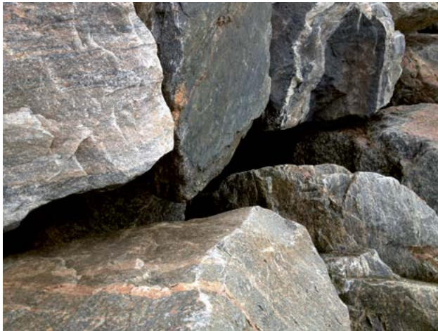
Figure 8-18 Example of failure in the underlayer, the breakwater/embankment is placed on filled materials, and subsidence and sinking into the underlayer cause the uppermost blocks to be hanging without good support. At the same time, the interlocking disappears that the overlying blocks should be providing for the blocks below. (Molde. Photo: Norconsult).
