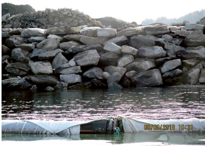
Figure 8-12 Example of breakwater/embankment with "structured rubble", see table 3-1. (Photo: Norconsult) The structure does not qualify as an interlocking surface because there are too many small blocks, the blocks are sitting with an incorrect slope and many blocks are sitting without support. MUST NOT BE USED IN BREAKWATER CONSTRUCTION.
