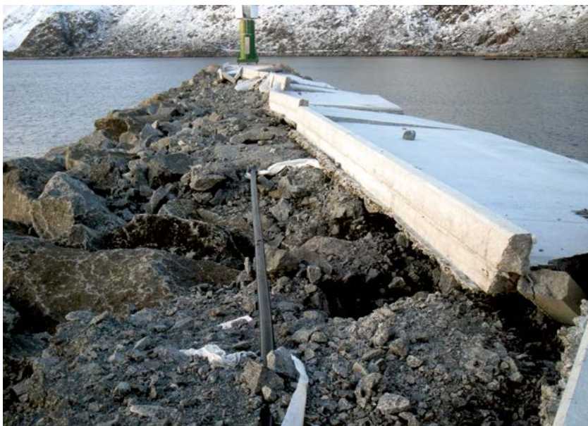
Figure 8-22 Example of lack of integration between deck and breakwater, where the crown wall is also absent. The deck is poured as a free-laying slab without the protection of a crown wall, and the deck is sitting on non-permeable material. During strong wave action with overtopping, the sea presses on the front edge, and the concrete slabs are lifted by the inner water pressure due to poor drainage. Note that the breakwater is otherwise undamaged. (Stamsund. Photo: Norconsult).
