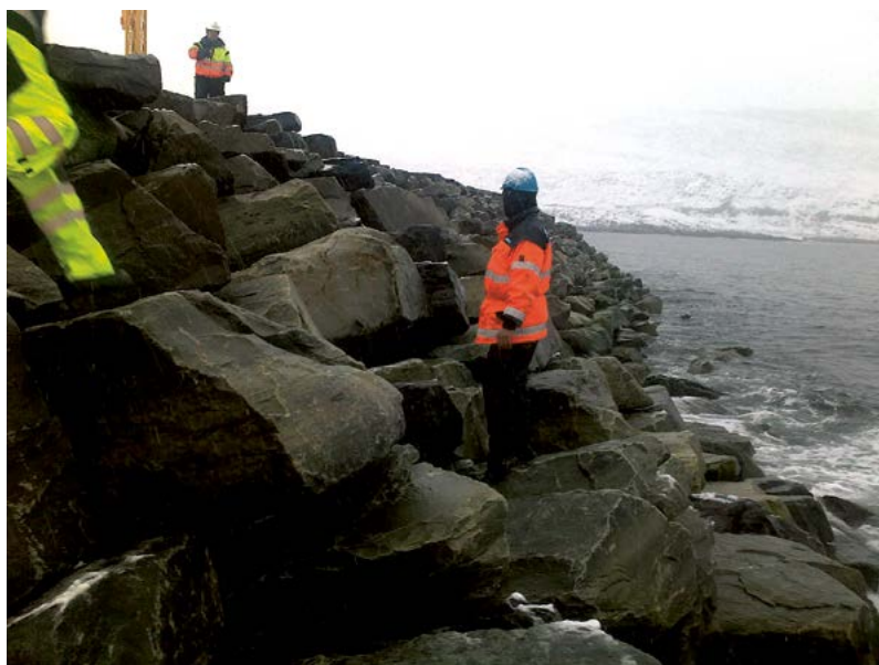
Figure 8-11 Example of a satisfactorily executed interlocking surface : The blocks are sitting interlocked with an acceptable slope, and are pointing weakly upwards. (Mehamn Airport. Photo: Norconsult).
