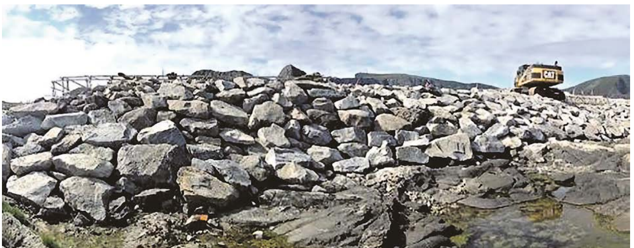
Figure 8-20 Examples of interlocking surface that has a low resistance capacity against high waves (but can be OK at less exposed locations): the blocks are sitting with an erroneous orientation, i.e. with the flat side in towards the breakwater. In this case, neither is the interlocking surface executed from the bottom up, and most of the blocks are sitting free without support. (Værøy. Photo: Norconsult).
