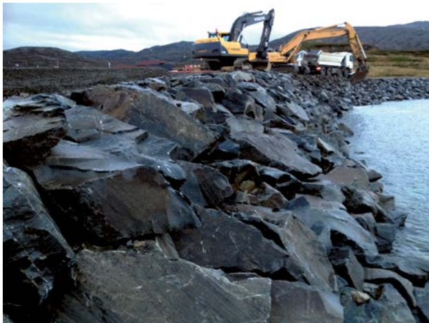
Figure 8-19 Example of interlocking surface that must be corrected: The blocks are partially sitting loose on the surface without support, and the blocks are sitting with an outward slope (pointing downwards). (Mehamn. Photo: Norconsult).
