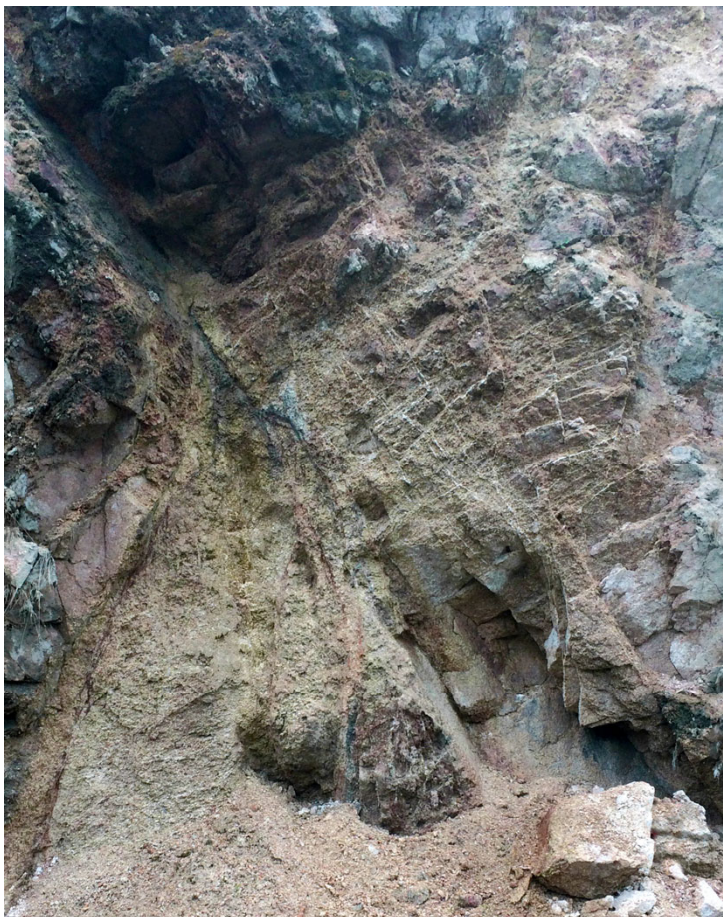
Fig. 11 Road cut just outside Drammen. This weakness zone crosses the Kleivene tunnel on highway E18
