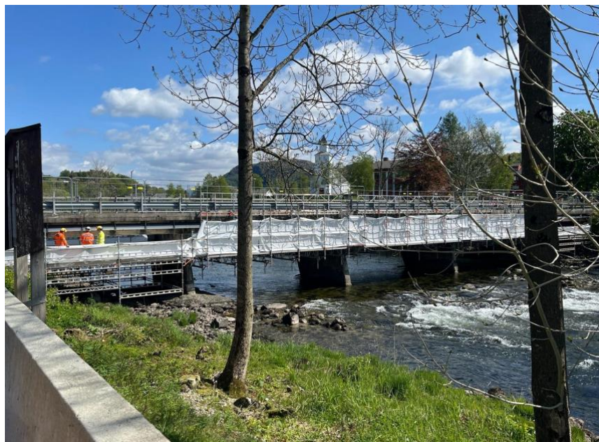
Figure 16: Photos of the riverbank at Bjerkreim segment A at the day of the survey (top), with large boulders and mounds of grass, metal scrap that could not be removed (middle), and the bridge by segment B under maintenance (bottom)
