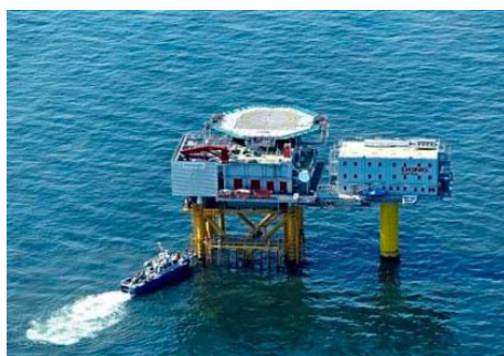
Figure 36. Offshore substation with accommodation platform alongside. Source: Dong Energy
