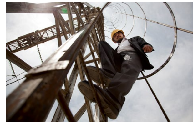
Network rehabilitation and expansion of electricity supply to Kabul, 2012. PHOTO: GRAHAM CROUCH/WORLD BANK
