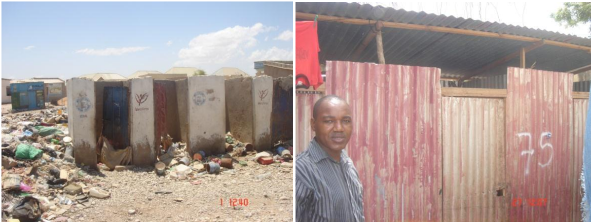
Figure 3 and 4: Non-NRC unmaintained latrines in Bossaso (left) and NRC well-maintained latrines in Mogadishu (right). Photo by A. Davies.
