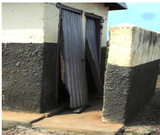
Figure 20: Toilet doors at Maper West. Photo J. Makongo.
