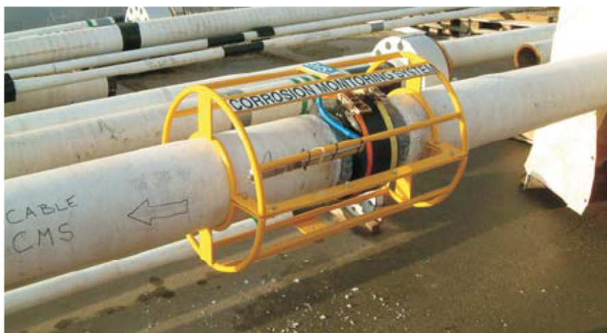
Figure 6.7: Guided wave sensor installed on pipeline (Evans 2007).
