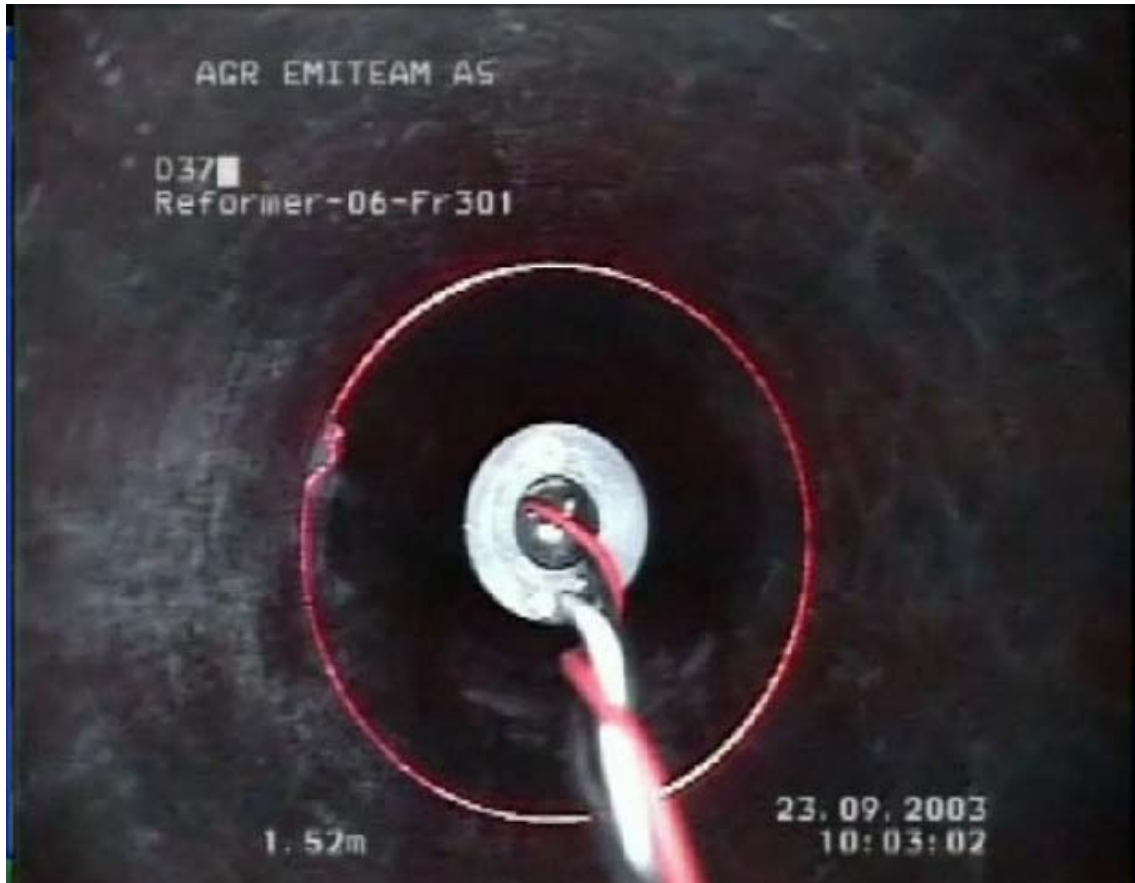
Figure 4.5 Screen capture from AGR promotional video on laser enhanced visual inspection. To the left an anomaly is clearly seen by the distortion of the laser ring (courtesy AGR Group)
