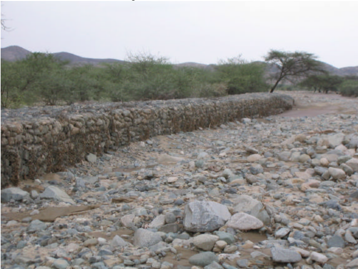
A newly constructed Gabion in Demas benefits target beneficiaries in Gahtelay to irrigate their plots of land distributed to rehabilitate them after they return back from the Sudan.
