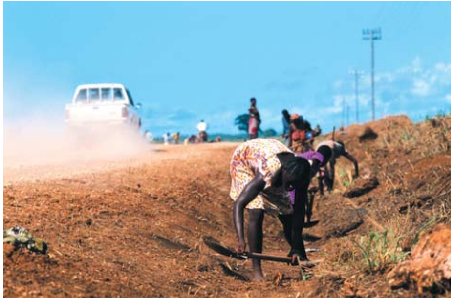
New, improved roads make necessary transport faster and easier. Norway has provided support for the road sector in Tanzania for four decades. Photo: Per Kristian Lunden
