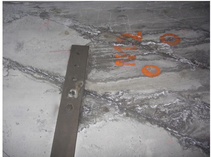
Abb. 4.1 Heavy cracks in the final lining
