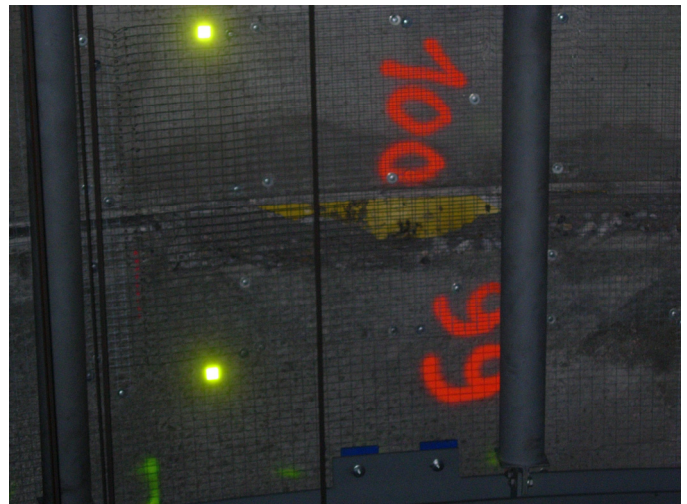
Abb. 4.2 Damaged sealing membrane in the upper part of the tunnel
