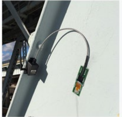
Figure 5-3 Picture of a wireless stain sensor mounted on a bridge /17/
