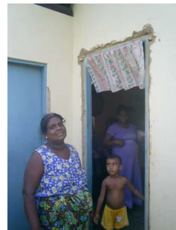
A houseowner show us how the doorframe is falling out on her new house in Hambantota.
