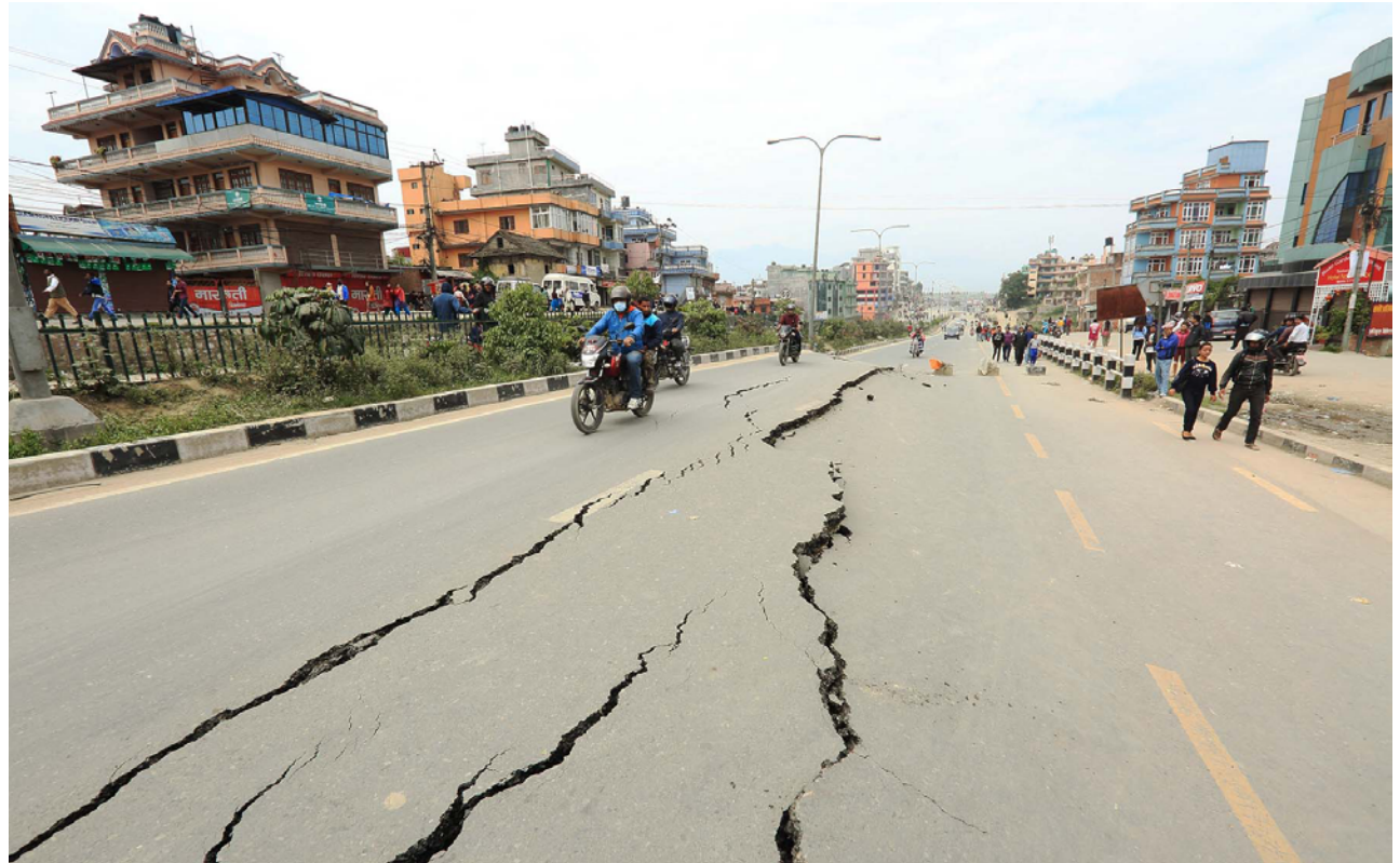
Earthquake damage in Bhaktapur, 2015. PHOTO: LAXMI PRASAD NGAKHUSI / UNDP NEPAL
