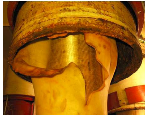
Figure 4-9 Blocked vent leading to breach in external cover, ref [12]
