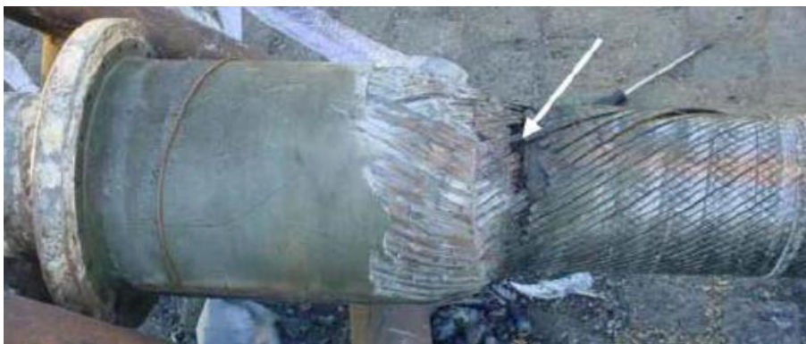
Figure 3-9 Severe armour wire corrosion / fatigue damage presented as Petrobras' experience, Ref [4]
