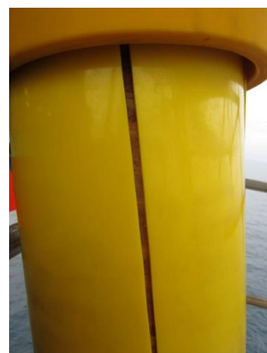
Figure 4-2 External sheath cracking
