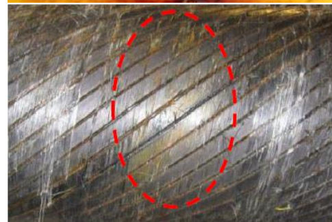
Figure 4-10 Typical external sheath cut with corrosion products on the surface, including wire inspection under the same damage, ref [28]
