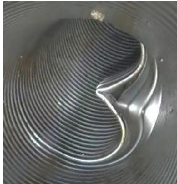
Figure 3-14 Typical small carcass collapse
